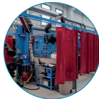
Manual welding stations for certified operators
